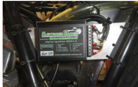
Figure 2 The ignition box is mounted in the frame on a piece of sheet metal.
