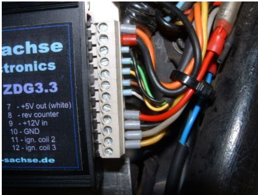
Figure 3 Mounting the ignition box and the terminal connector.
